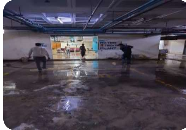
Reverse bleeding of grout from floor.
